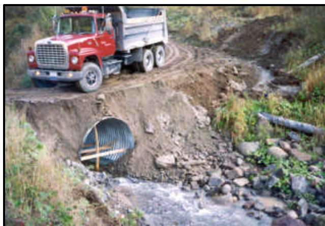
Water crossing structure creating erosion (source : MRNF)
